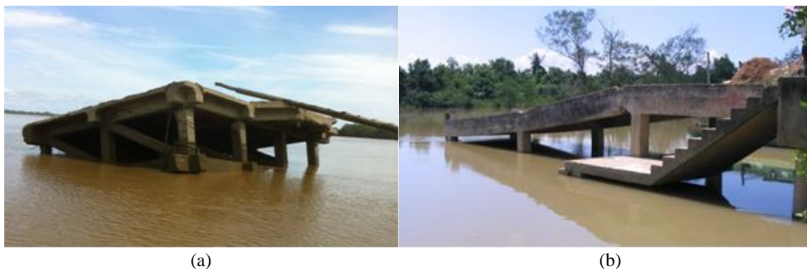
Figure 1 Failure of (a) wharf at the Lupar River and (b) jetty at Kpg. Hulu, Samarahan Division [1]-[2]
