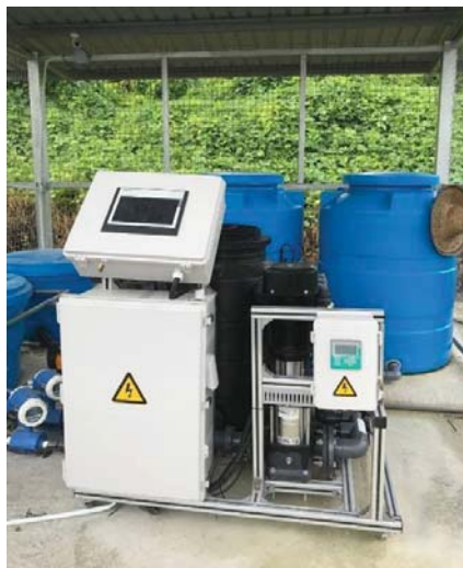
Figure 2.8 Automated fertigation system to control fertilizer content and irrigation and storage tanks. (Photo taken at Agriculture Research Centre, Semongok.)
