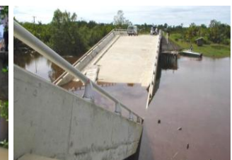
Fig. 4: Collapsed Sg. Palasan Bridge in Betong Division
