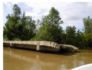
Fig. 1: Remains of collapsed wharf at Sg. Saribas
