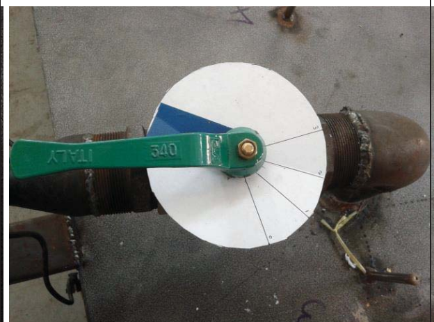
Figure L 76: Air flow rate level indicator at blower 2
