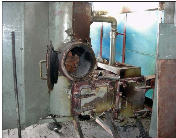
Figure 1.14: Main body of B2E converter broke open/through after 3 months into operation
