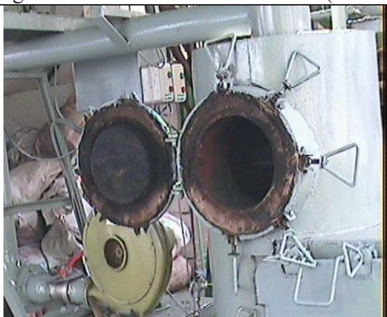
Figure 1.7: A view of B2E pyrolysis chamber
