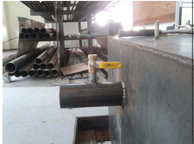
Figure L 68: A ball valve pipe is installed at the middle of the exhaust for flue gas measurement
