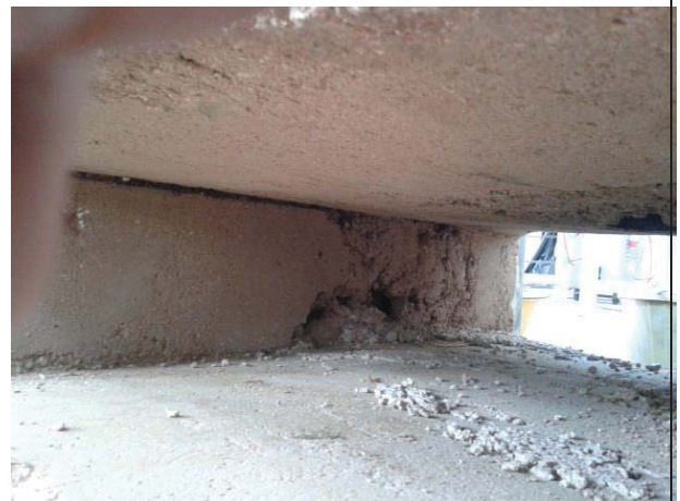
Figure L 28: Void formed inside the tar removal chamber
