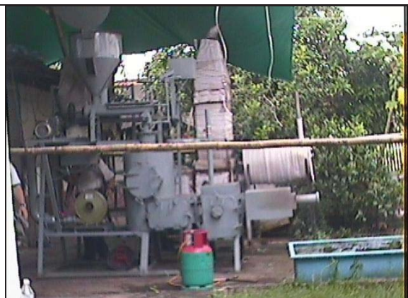
Figure 1.5: A view of B2E converter (Onsite)
