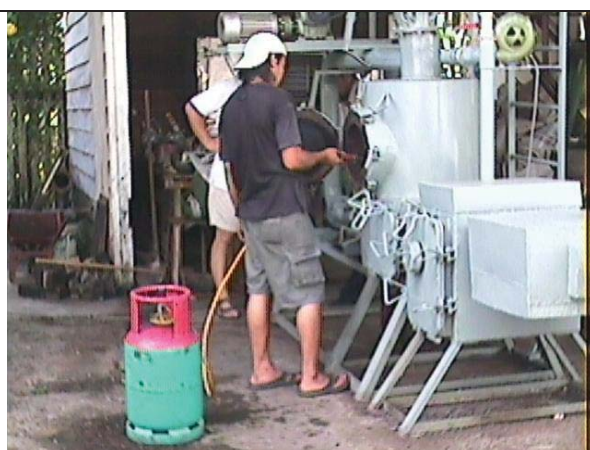
Figure 1.13: Initial ignition of feedstock in pyrolysis chamber
