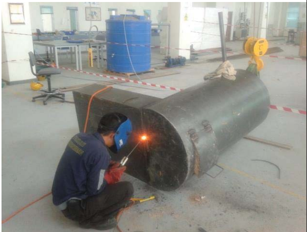
Figure L 49: Welding pyrolysis chamber and tar removal chamber (holding by overhead crane)
