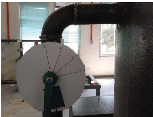
Figure L 75: Air flow rate level indicator at blower 1
