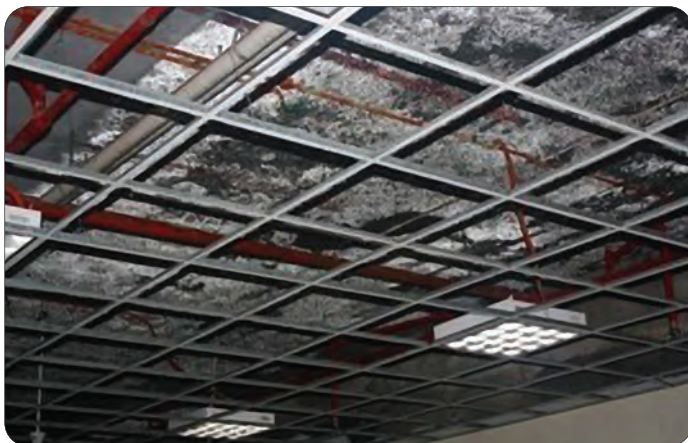
Figure 4. Condensation on the soffit of a RC slab.
