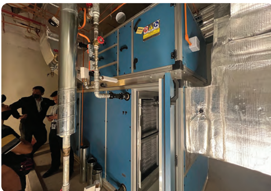
Figure 5. A retrofit project involving the installation of a new Air Handling Unit (AHU).
