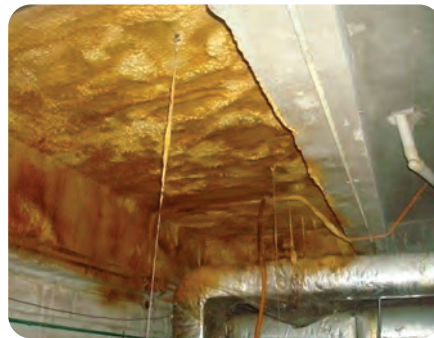
Figure 3. Wet and saturated PU foam.
