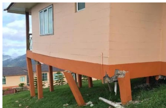
Fig. 2 - Stilt house damaged due to short column effect
