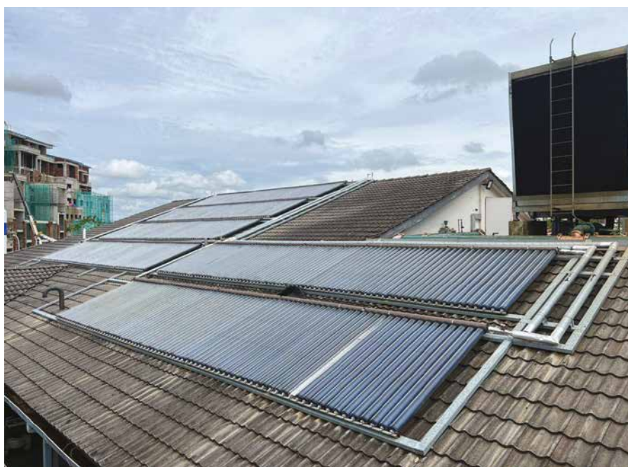
Figure 5: The solar thermal hot water supply system at Hospital Miri Sarawak.
