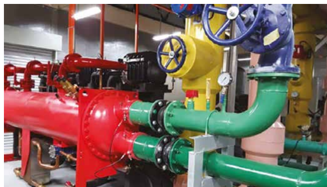
Figure 4: A chiller retrofit at Hospital Teluk Intan involved applying variable-speed, oil-free centrifugal chillers with magnetic bearings.
