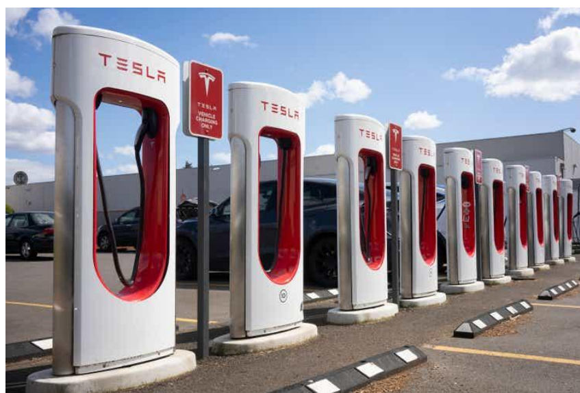
Figure 2.1: Tesla's Supercharger Station
