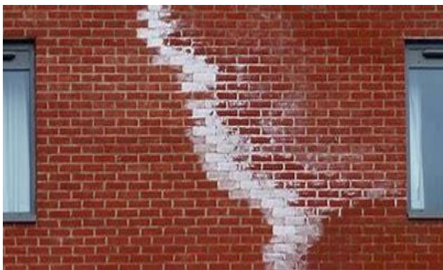
Figure 2.4 Efflorescence damage on brick wall.
