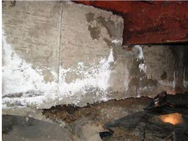
Figure 2.2 Efflorescence damage on concrete wall.
