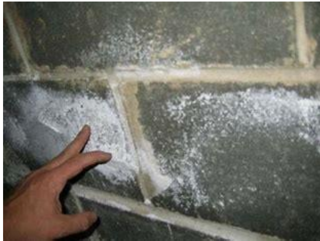
Figure 2.3 Efflorescence damage on brick wall.
