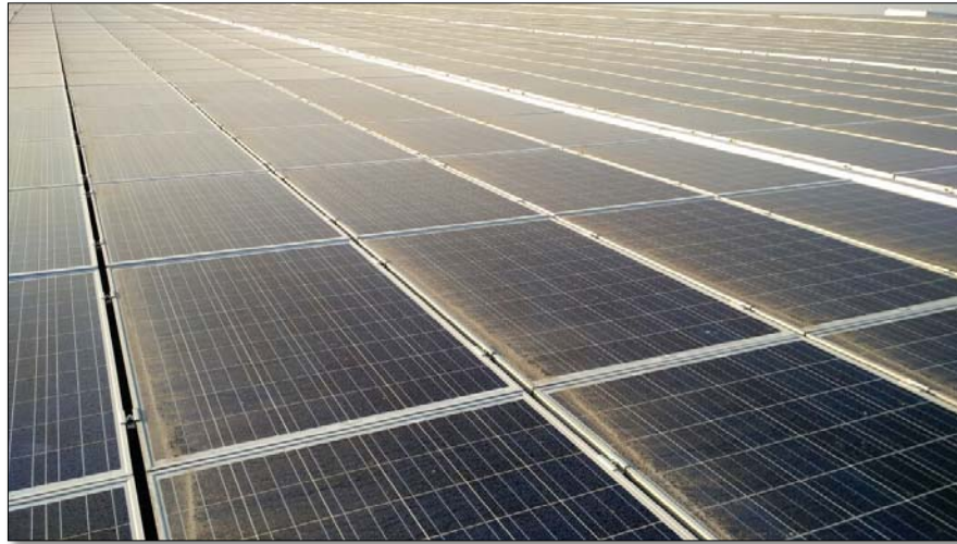
Figure 1.1: Solar Panels with dust accumulation [4]
