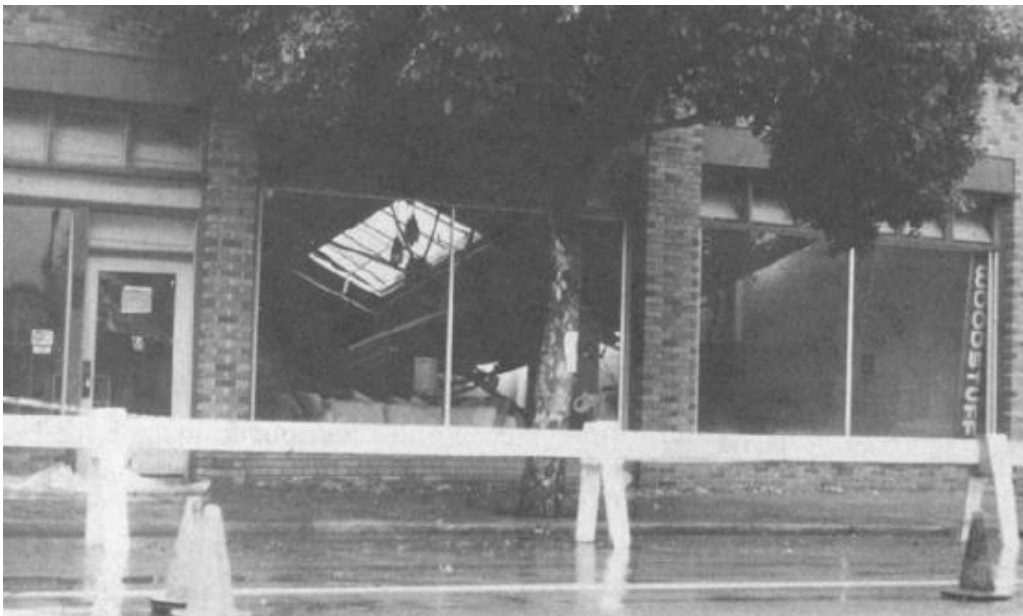
Figure 1.2: Typical Failure of Slipped Roof Joists Off Their Wall Supports (Bruneau, 1994)
