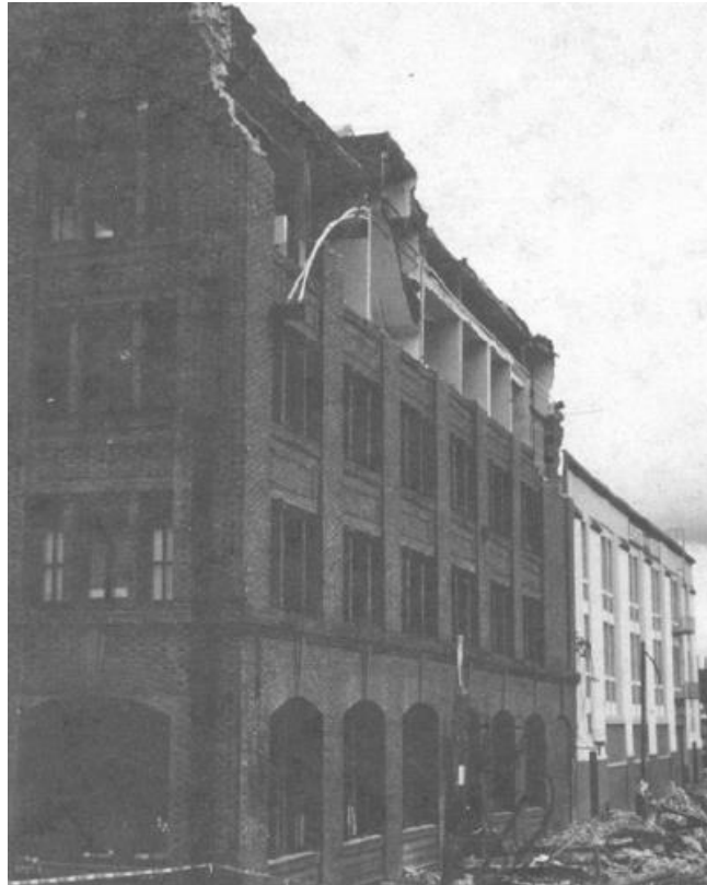
Figure 1.3: Out-Of-Plane Failure of URM Top-Storey Wall at San Francisco, Loma Prieta Earthquake (Bruneau, 1994)
