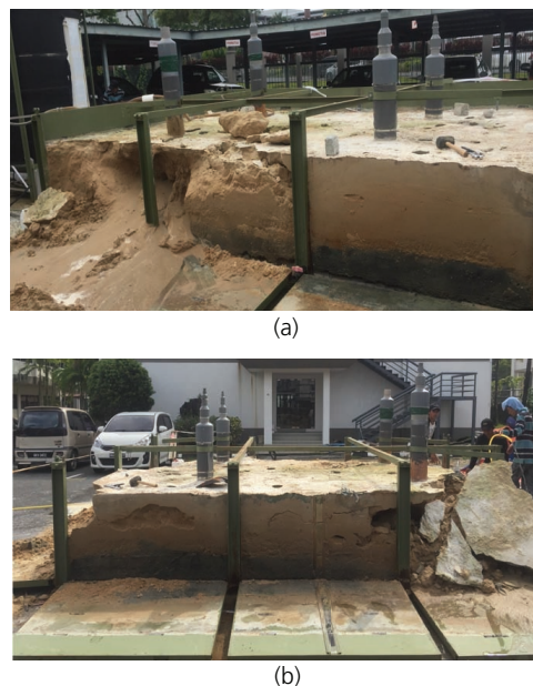
Figure 1. A sandbox ( 10 \text{ m}^3 ) was subjected to bio-cementation treatment. (a) Front view of the treated soil mass after an outdoor trial treatment; (b) rear view of the treated soil mass
