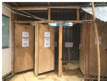
Fig. 7. Construction Site C workers' quarters' utility cables hanging lowly across the quarters.
