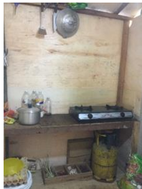
Fig. 3. Construction Site A makeshift workers' quarters kitchen where there is a pose of fire hazard
