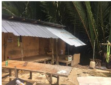
Fig. 6. Construction Site C workers' quarters sited on the corner of the construction site.
