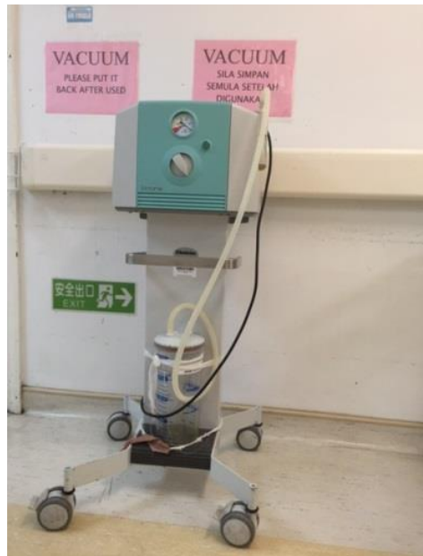
Vacuum pump machine
