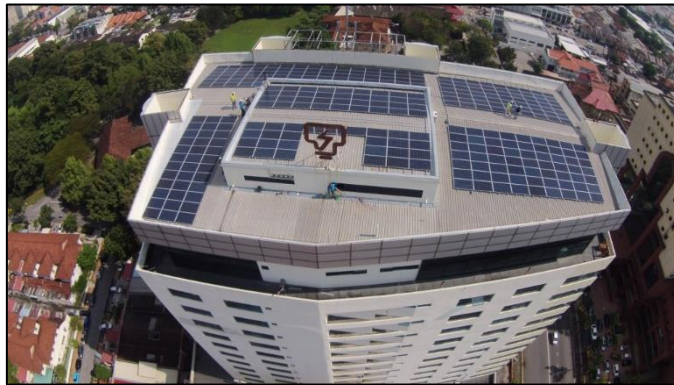
Figure 1.4: Rooftop solar PV in TNB building [12].
