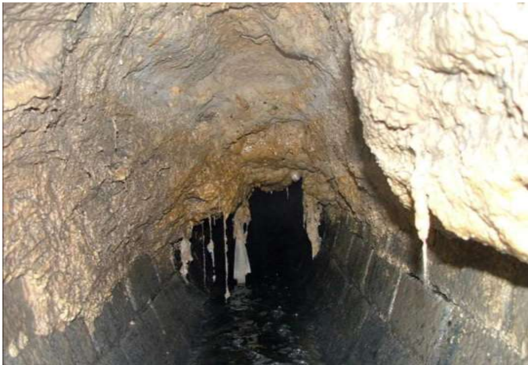
Figure 2.2. FOG deposition in sewer pipelines. (Adapted from Kolev Slavov, 2017).
