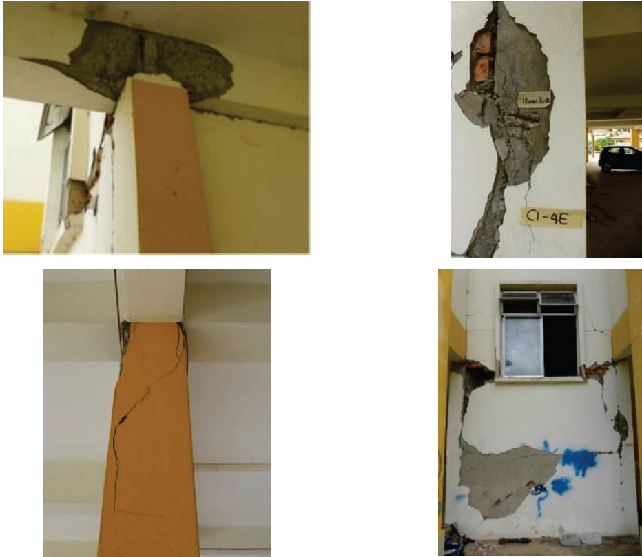
Figure 2.2: Crack on Column and Wall at Ranau School
