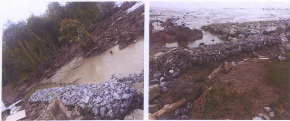
Figure 1.2: Gabion Wall before and after wave hit at Kampung Serpan Laut, Asajaya
