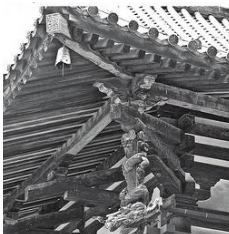
Figure 1: Bracket system that is used to hold the timber beam of Horyuji Temple
