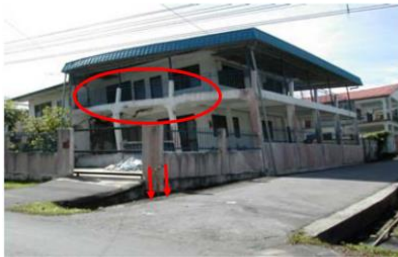
Figure 1.4. Ground subsidence at housing area in Sibul town. (Duraisamy, Huat, & Aziz, 2007)
