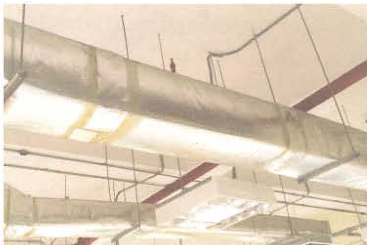
Figure 7: Squared metal sheet insulated fiber glass ducting board installations roof top unit
